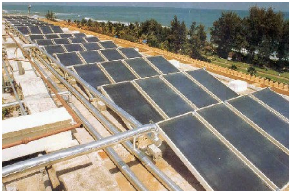
Figure 5.2 Solar water heating system for hotel (capacity 20000 lit /day)
