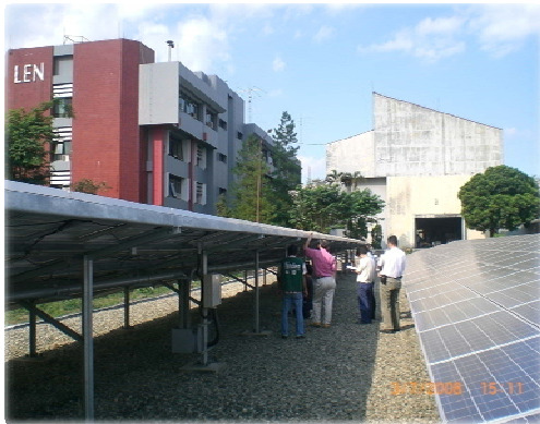
Figure 7.3. 80 kW p Solar Panel in Bandung (Source : DEMR)
