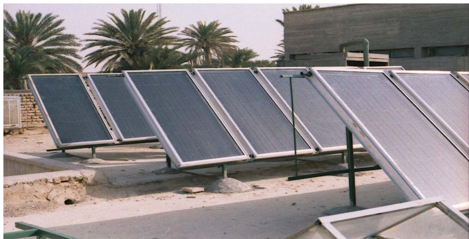
Fig.8.26 Solar collectors for Mosala of Zabol
