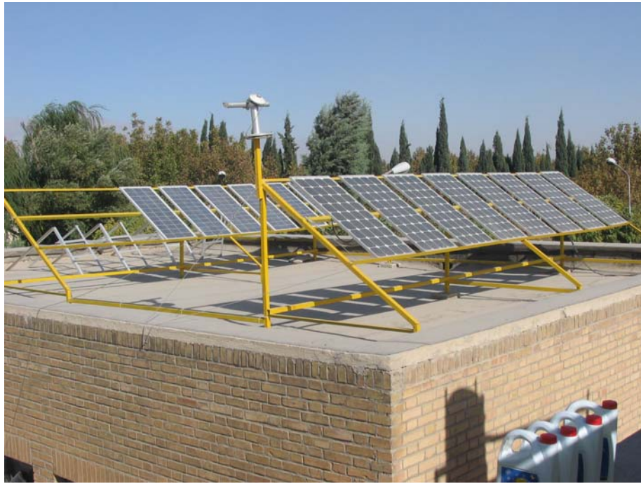
Fig.8.3 Photovoltaic for producing electricity (3 KW)
