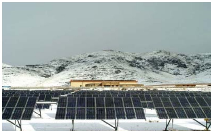
Fig.4.12 Design and installation of grid connected and off-grid photovoltaic system In different area with total capacity 175 KW (2002-2004)
