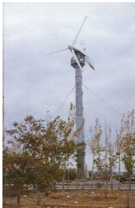
Fig.4 17 Ten KW e unit for a village near Tabriz
