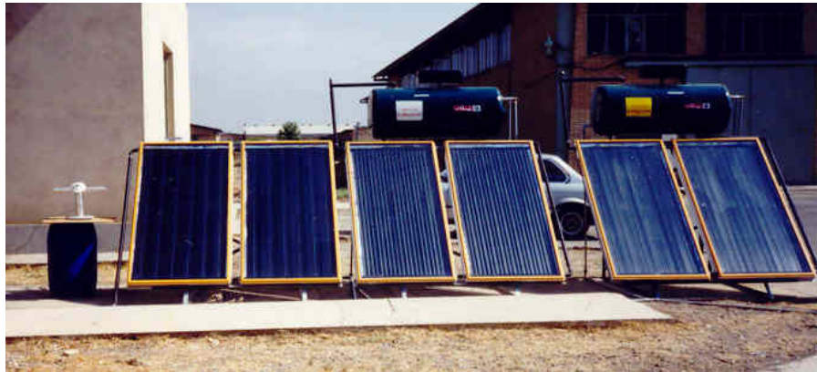
Fig.8.9 Collectors under test
