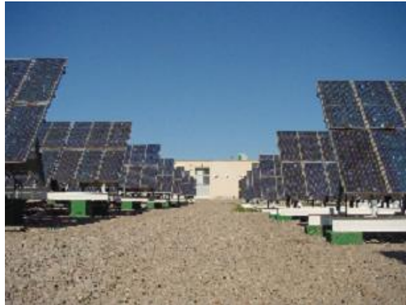
Fig.4.10 Semnan area with 97 KW e
