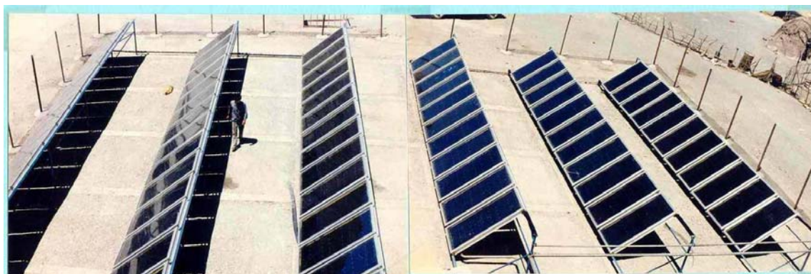
Fig.8.16 Side view of solar collectors
