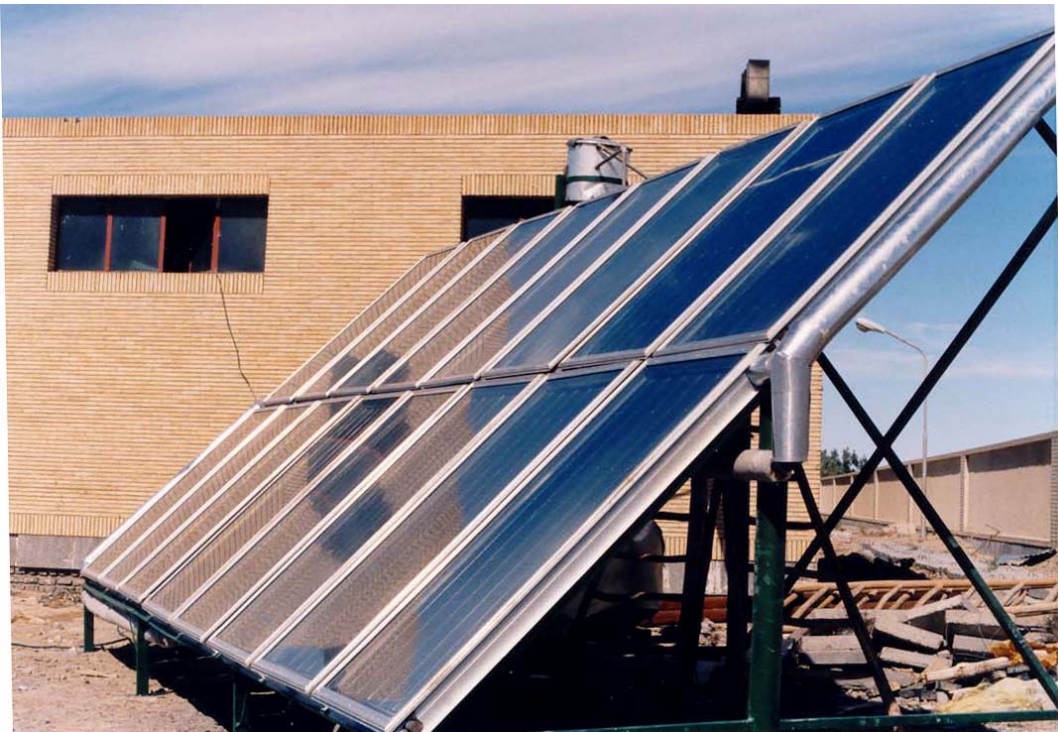
Fig.8.11 Solar Collectors and storage tanks under the structure
