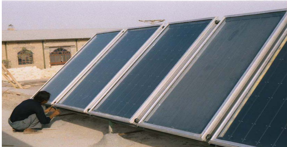
Fig.8.27 Solar collectors for Mosala of Zahak
