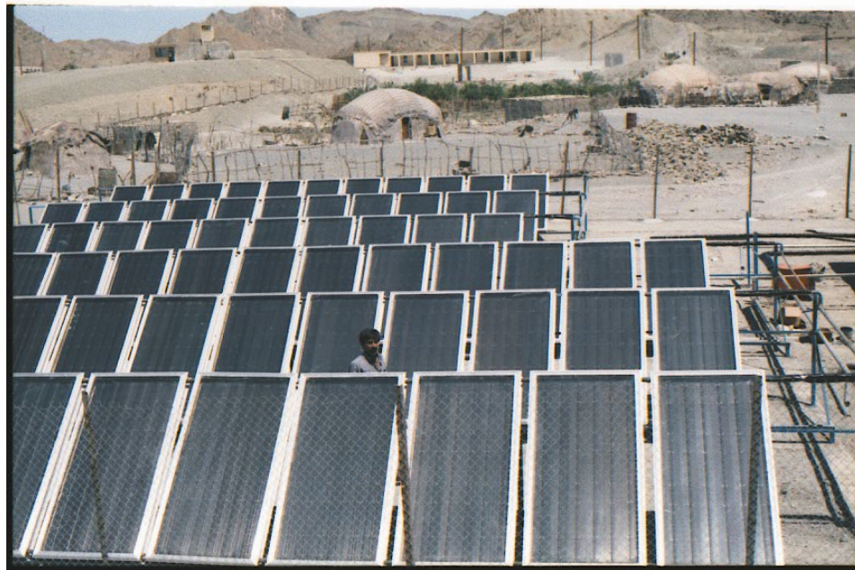
Fig.8.15 Front view of solar collectors
