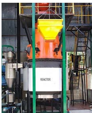
Figure 2.2 – EnerFab Thermal Gasifier
