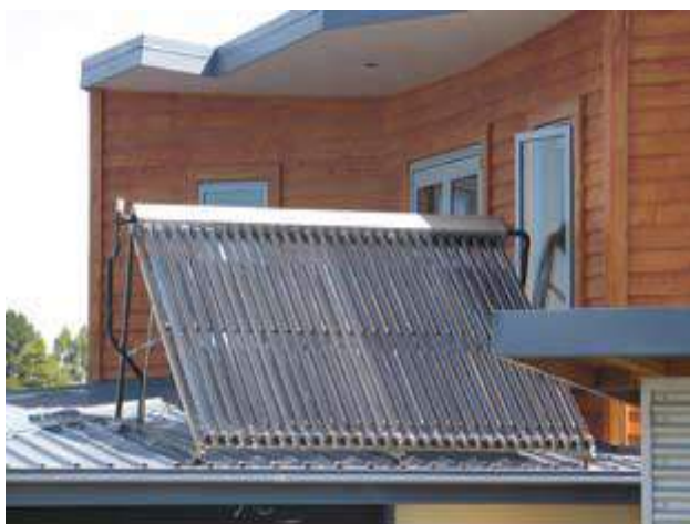
The roof-top solar collector
