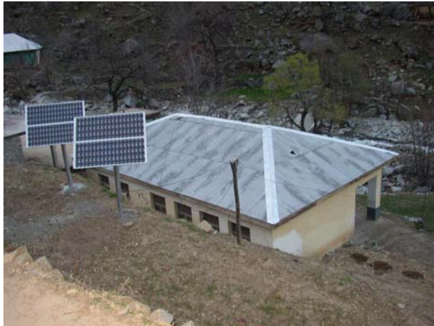
400 Watts Solar Lighting System Installed at School of Remote Area of Pakistan
