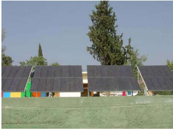
Solar Powered System at Jalalabad Park Azad Kashmir, Pakistan
