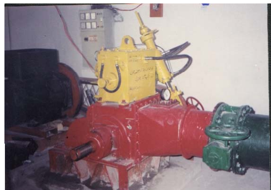
A Microhydel Plant installed in Tribal Areas of Pakistan
