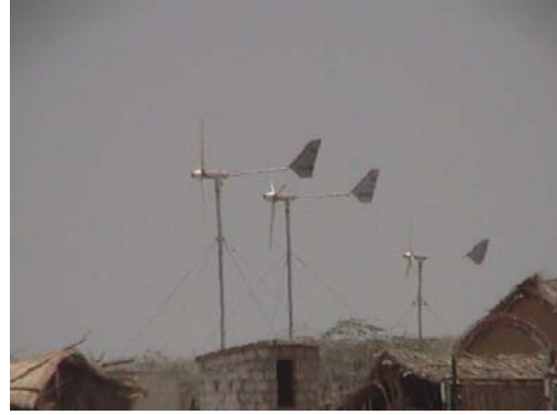
Micro Wind Turbine Installed at Coastal area of Pakistan
