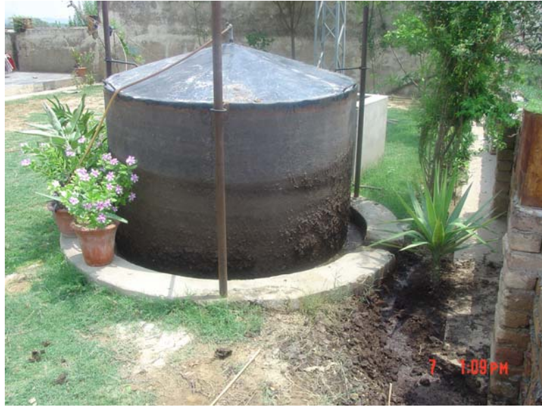
Biogas Plants Five Cubic Meters Capacity
