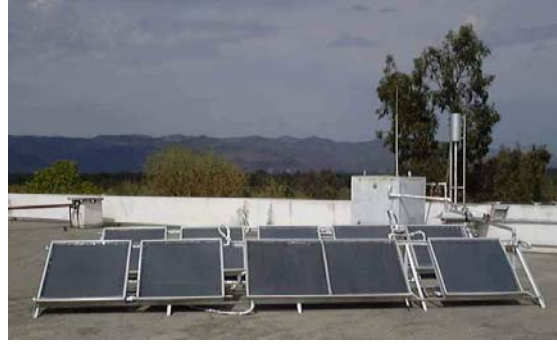
Solar Water Heating System for Space Heating
